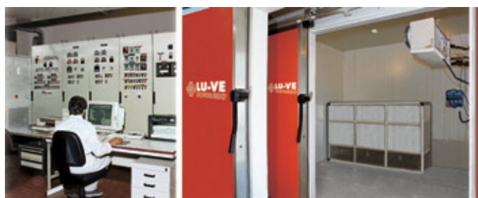
Dooble cold rooms laboratory
